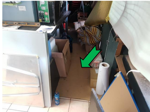
Photo 10. Interior, central south elevation, bar area, floor – non asbestos containing vinyl sheet and adhesive.
