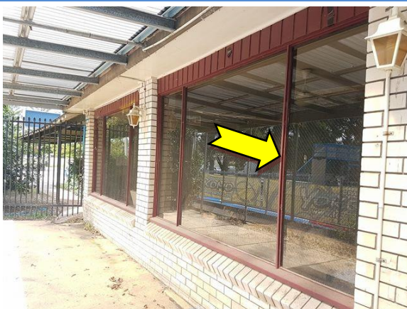
Photo 17. Exterior, throughout, windows and door frames – suspected lead-containing red upper coloured paint system.
