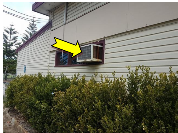
Photo 24. Exterior, throughout, air conditioning units, refrigerant R22 – ozone depleting substance.
