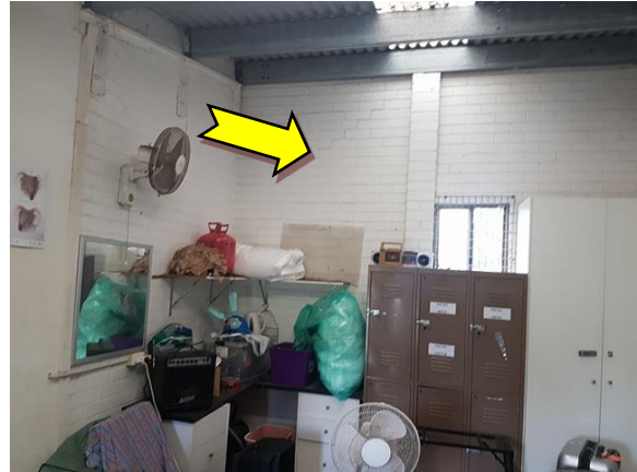
Photo 20. Interior, south-east elevation, garage, walls – suspected lead containing white upper coloured paint system.
