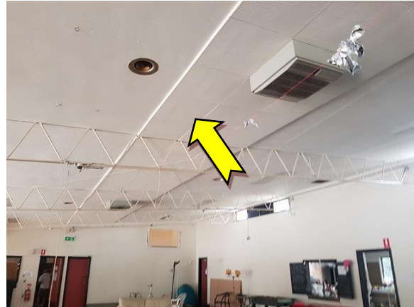
Photo 14. Interior, main hall, ceiling – suspected SMF-containing compressed ceiling tiles.
