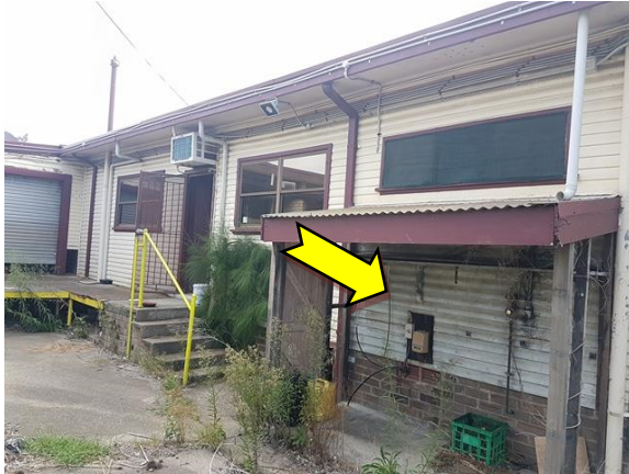
Photo 19. Exterior, throughout, walls – suspected lead-containing cream upper coloured paint system.
