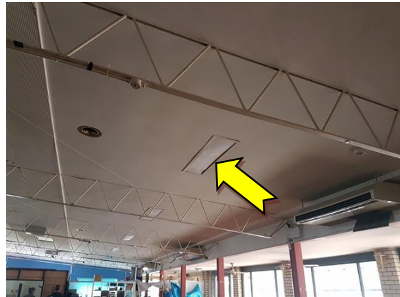
Photo 16. Interior, throughout, double tube fluorescent light fittings – suspected PCB-containing capacitors.
