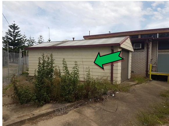
Photo 4. Exterior, central east garage, walls – no materials suspected of containing asbestos identified. Materials formed of masonite.
