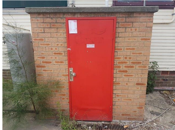
Photo 26. Exterior, north-east elevation, electrical switch room – no access at time of assessment due to locked door.
