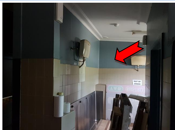
Photo 6. Interior, north-east elevation, toilet walls – asbestos-containing fibre cement sheeting.
