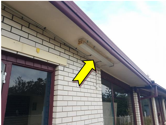
Photo 15. Exterior, throughout, double tube fluorescent light fittings – suspected PCB-containing capacitors.
