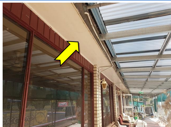
Photo 18. Exterior, throughout, eaves – suspected lead-containing cream upper coloured paint system.
