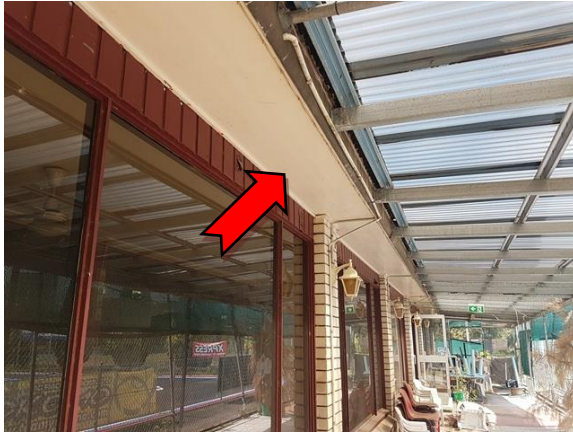
Photo 1. Exterior, throughout, eave lining – asbestos containing fibre cement sheeting.
