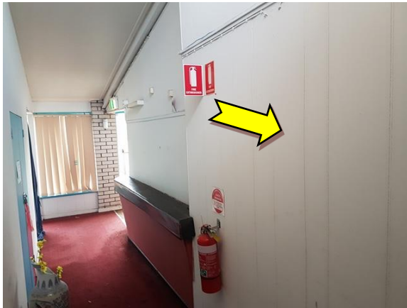
Photo 21. Interior, throughout, walls – suspected lead containing white upper coloured paint system.
