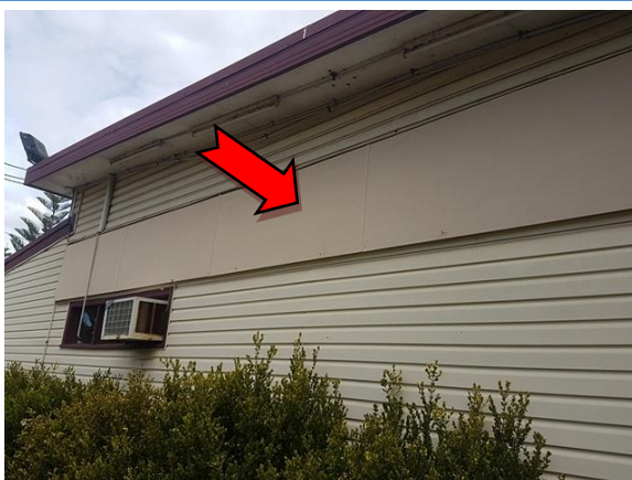
Photo 5. Exterior, north elevation, façade – suspected asbestos-containing fibre cement sheeting.
