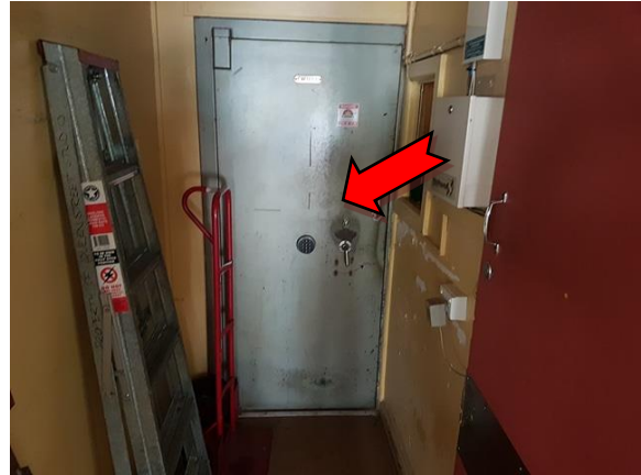
Photo 8. Interior, central east elevation, security room, door – suspected asbestos-containing internal insulation.
