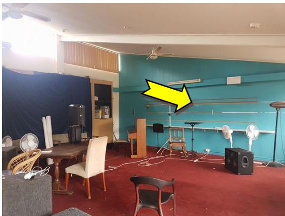
Photo 23. Interior, central east elevation, walls – suspected lead containing blue upper coloured paint system.
